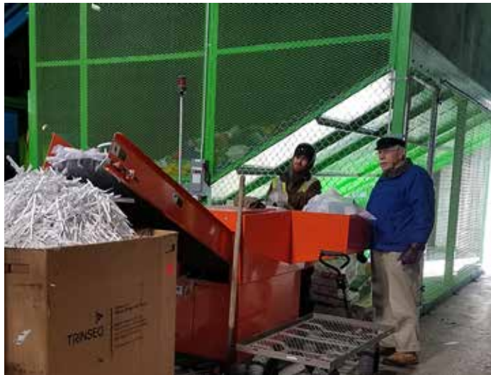
Fencing the area behind our shredder (green above) and surveillance cameras now allow ECR to secure documents for later shredding.
